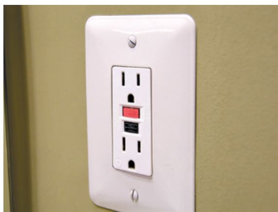
PHOTO: GFCI outlets are safer than other types of outlets in wet areas.
