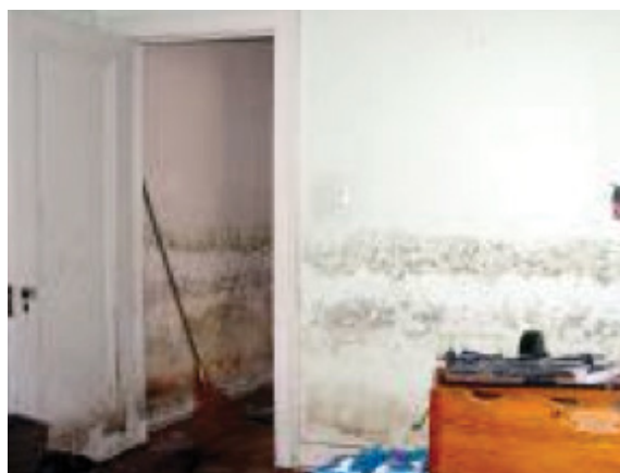
PHOTO: Mold growth in flooded home.
