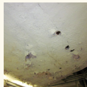
PHOTO 2: Ceiling damage resulting from roof leaks.
