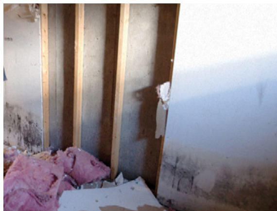
PHOTO: Remove all wet or fire-damaged insulation, even if wallboard appears to have dried.
