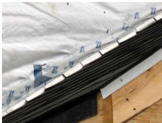
PHOTO: A water-resistant barrier layered over step flashing at a roof-to-wall intersection.
